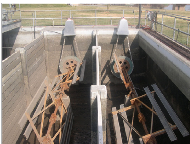
Figure 5. Flocculation chamber of basin 1.
